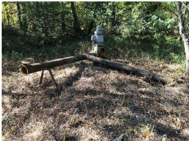
Photo 12. Well pump (photo courtesy of MVS-USACE).
