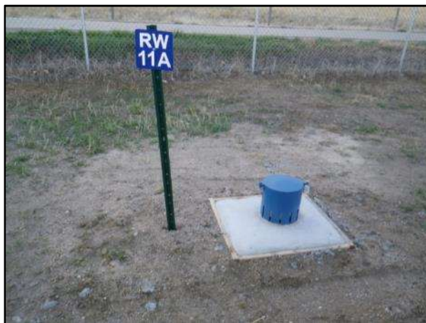
Photo 6. Relief well (photo courtesy of NWO-USACE).
